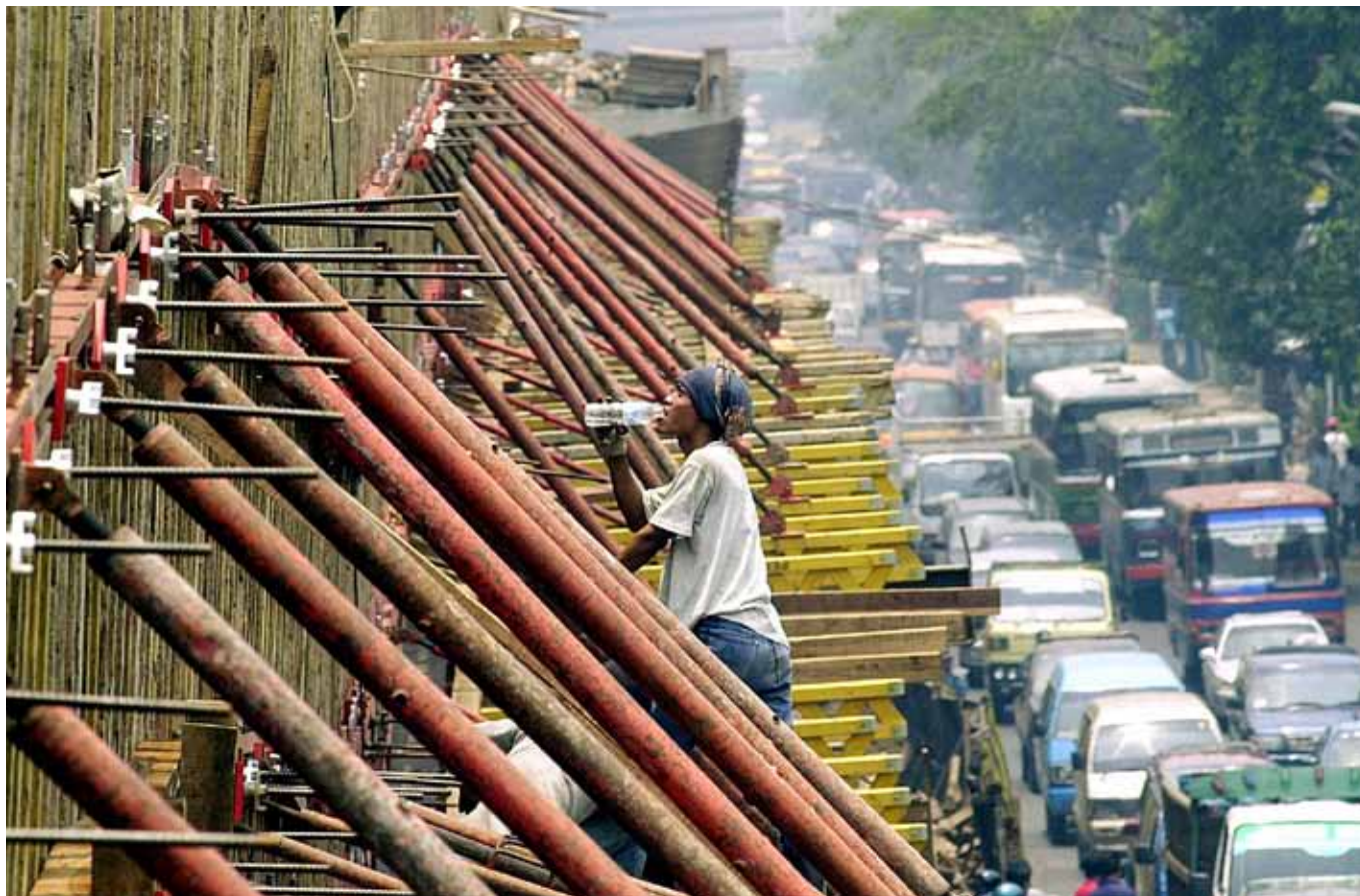
A bridge under construction in Jakarta: Indonesia has made major efforts to increase efficiency in public procurement processes.
